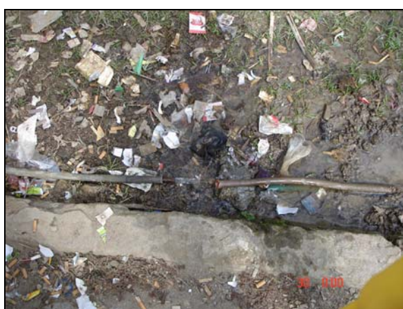
Picture 6: Water pipe from the mountain to household: it's broken and that makes the water contaminated.
