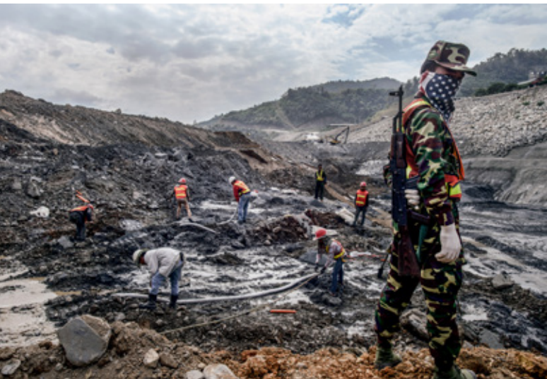
A Lao soldier is guarding construction workers while they are exploding the rock in front of the dam with flash powder Photo: Jittrapon Kaicome
