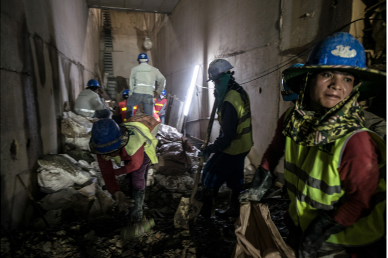
Construction workers are working inside the tunnel of the navigation lock. / Photo: Jittrapon Kaicome
